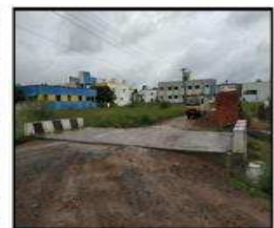
Construction of RCC slab culvert of vent 1.50m (3 Numbers) in Ravappa Nagar at Varadarajapuram Panchayat
