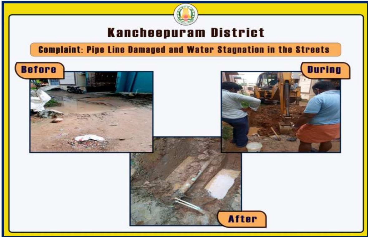
Twitter Complaint Subject: To restore damaged Pipeline
