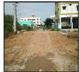
Construction of 2 Nos. of RCC slab culvert of vent 2.00m at Balajinagar at Varadarajapuram Panchayat
